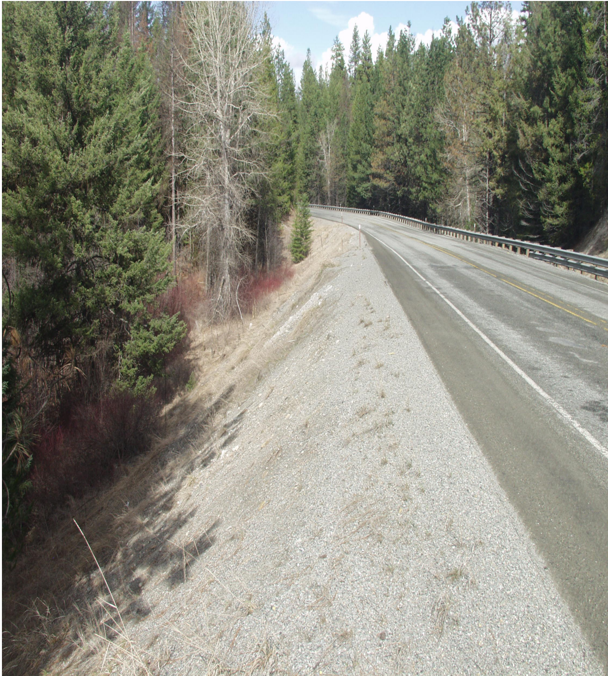
Photo 14: State Route 155 Lack of Guard Rails 2015
